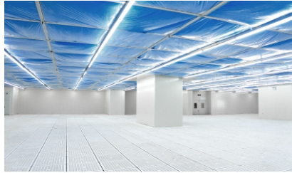
光学百级洁净室 Optical hundred clean room.
