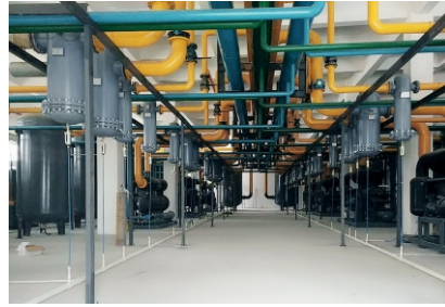
空压站 Air pressure station.
